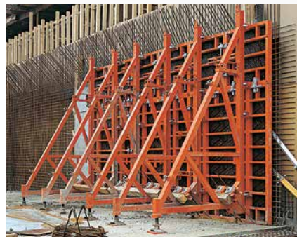
SB-B and SB-C Brace Frame units with TRIO Panel Formwork with a concreting height of 3.50m.
