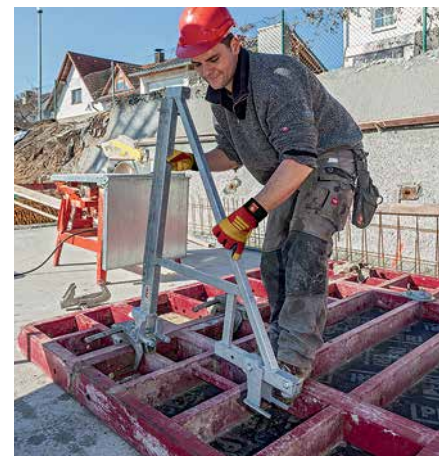
The working platforms are mounted on the element of the corresponding width and also remain attached to the formwork during temporary storage.
