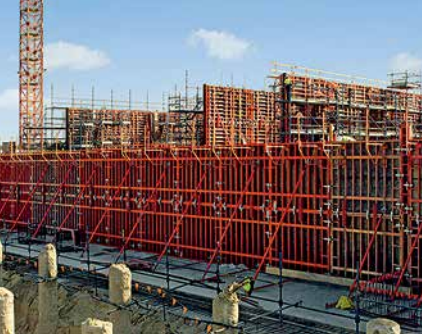
Kurnell Desalination Plant, Sydney, Australia
