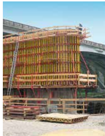
Sides of hollow piers on the banks of the river, climbed with VARIO GT 24 on PERI KG 240 climbing scaffold. Adapting to the arch-shaped ends was achieved with VARIO standard components and forming boards.
