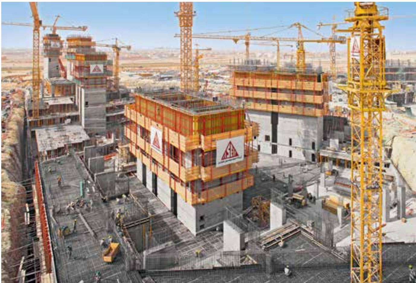
VARIO GT 24 on the RCS rail climbing system for constructing the elevator and stairway shafts of a highrise building.
