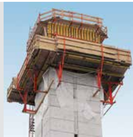
Church steeple in Feldmoching near Munich. VARIO GT 24 on KGF 240 climbing formwork.
