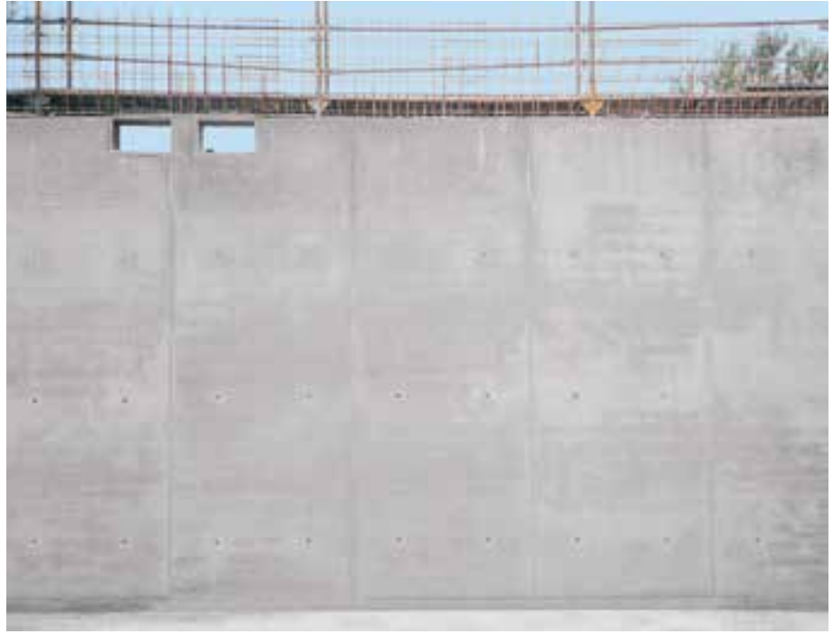
An orderly pattern of ties spaced at 0.75 x 1.18 m and smooth, architectural concrete are the result (Secondary School in Kletov).
