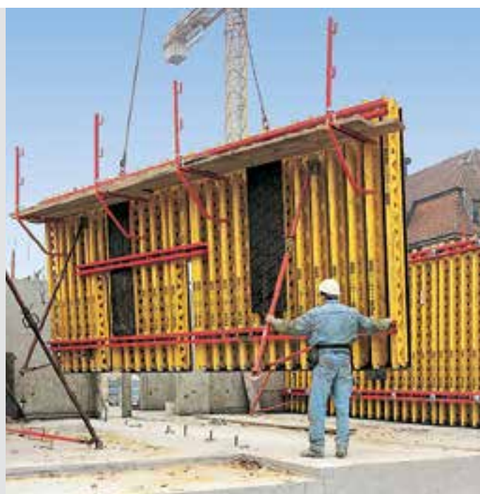
Soundproof sealing of the tie points costs 50% less as the top tie point is above the concrete with a spacing of 2.37 m.
