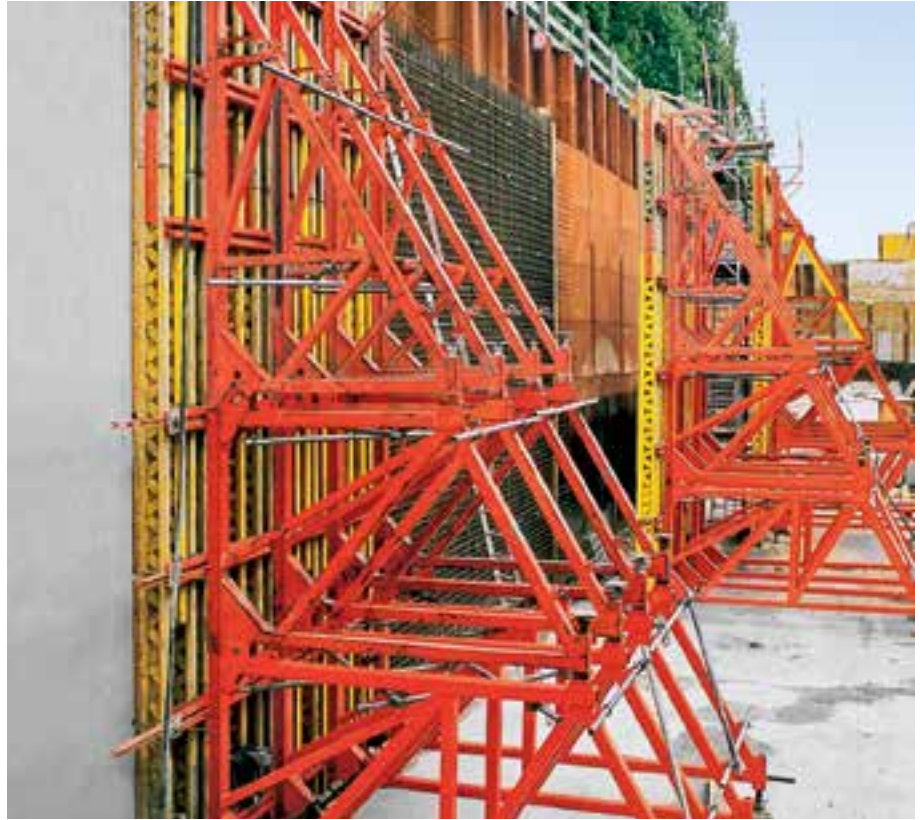
Max. concreting height of 8.75 m, Brace Frame SB-A0, A, B and C with VARIO GT 24 wall formwork.
