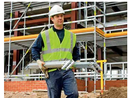
The small width of the UH Ledger allows up to 4 ledgers to be carried at any one time by one scaffolder.
