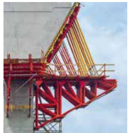
The spacing and number of Brace Frame Sections are determined through the existing load.
